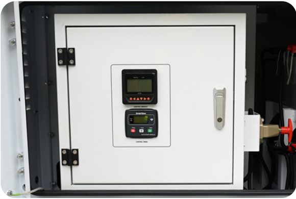
Distribution / Conversion panel
